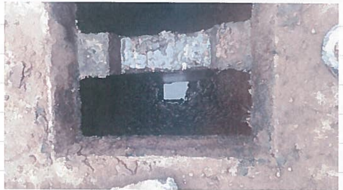
MIDDLE BAFFLE WALL; SOLID SEWAGE IN OUTLET COMPARTMENT OF TANK
