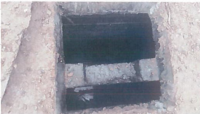
INLET COMPARTMENT MOSTLY EMPTY ~1 INCH WATER
